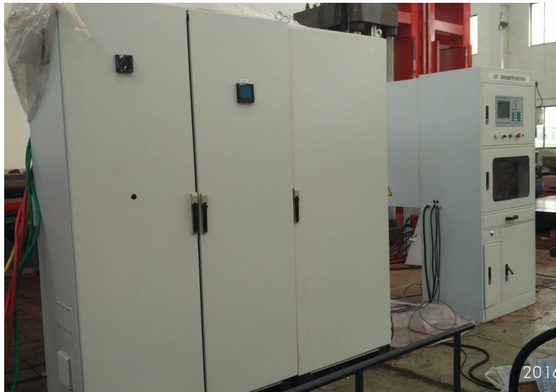
Electrical Control Cabinet & Operation Cabinet for Hydraulic Power Unit
